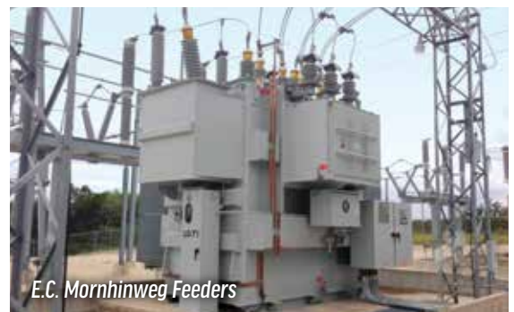
Hueco Springs Substation and Feeders
