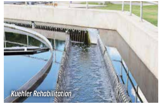
McKenzie Water Reclamation Facility
