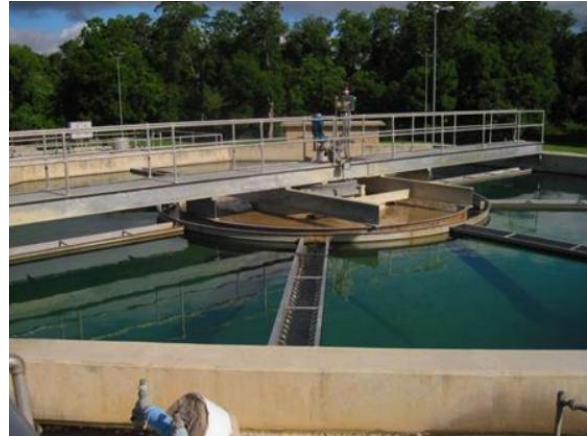
Figure 2-1: SWTP Upflow Clarifiers
